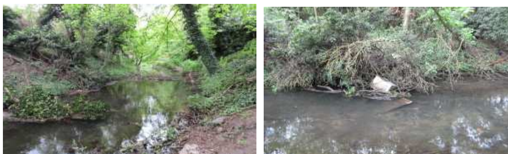
Rubbish in channel
